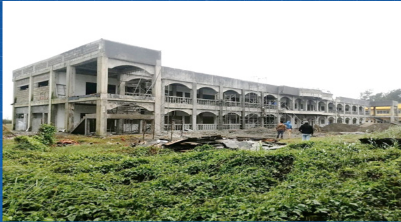
CONSTRUCTION OF SCHOOL BUILDING IN THE COLLEGE OF FISHERIES FOR LABORATORY RESEARCH AND DEVELOPMENT Percentage Completed: 84.77%
